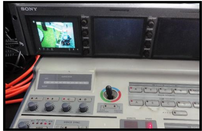
Fig. 17 Photogram sent from the IU to the monitors located in the premises of the central building
